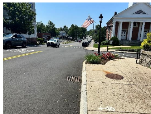
Image 7: Uncontrolled crossing across both Central Street and Essex Street missing pedestrian signage.
