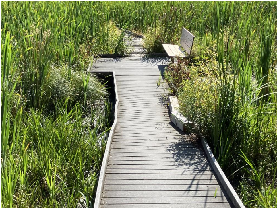
Mary French boardwalk, right side sinking into the marsh.
