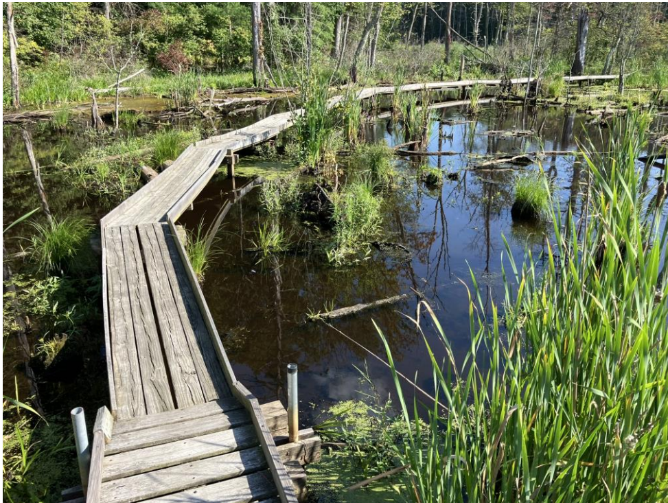
End section of boardwalk where the decking is beginning to warp and buckle due to water damage and use. During the wet season, the water comes within three inches of overtopping the boardwalk.
